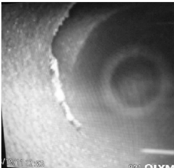
图 14 内窥镜观察缺陷状态 Fig.14 Defect state observation by endoscope
